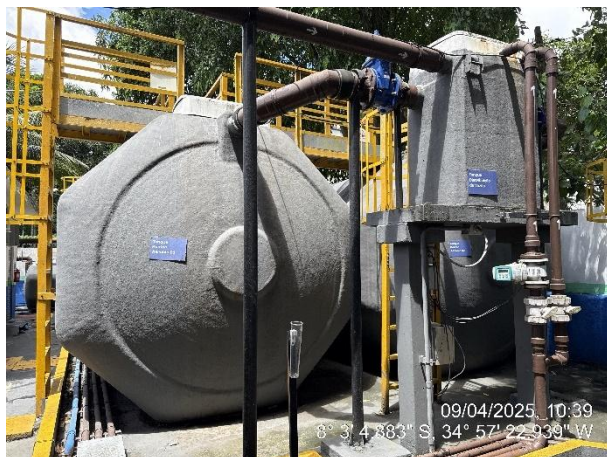
Tanque reator aeróbio
